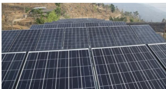
Solar panels installed on rooftop and ground at Kaduwa village in Khotang district. Post (File photo)
