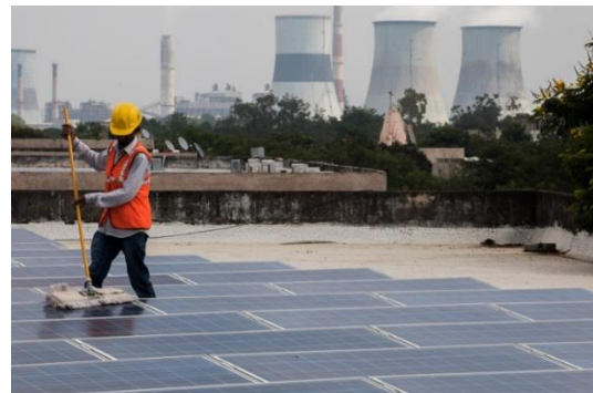
Solar panels installed on the roof top of the government building in Gandhinagar contrast with a neighboring coal-fired power plant.
