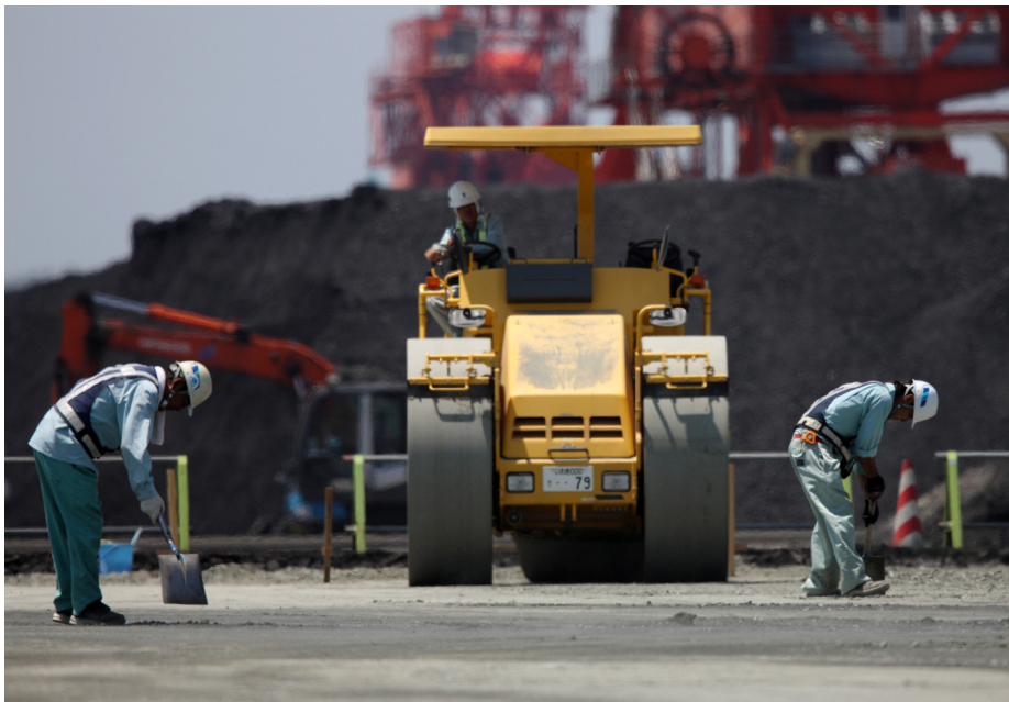
Workers repair a coal loading facility at Onahama port in Iwaki, Fukushima Prefecture. Japan's government and industry are backing emerging coal technologies that they say are less damaging to the environment. Bloomberg
